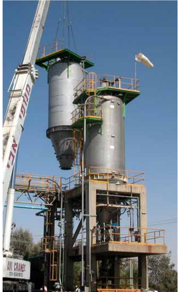
Installation of two VRM mixers for the handling of fungicide
